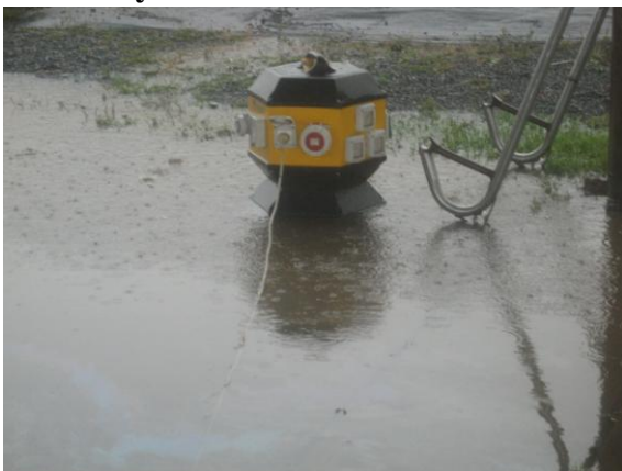
This was under the pit roof ...
